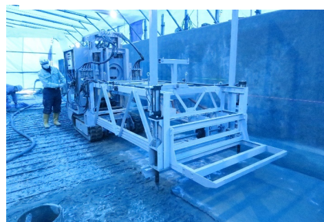
Fig.4 水路底版部での機械化施工 Applying an automatic trowel machine for a drain slab.
