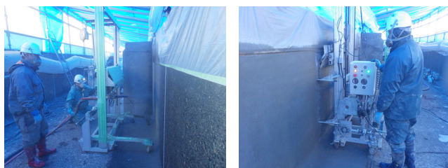
Fig.2 従来工法と機械化施工の比較 Comparisons between conventional and mechanical procedures
